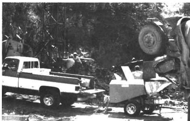
Cementing operations at Monticello Oil Co. Ltd. well No. 2, classified as hazardous by the California Division of Oil and Gas. The cementing operations are part of a procedure undertaken to properly abandon the well. Photo by Ed Hickey.
