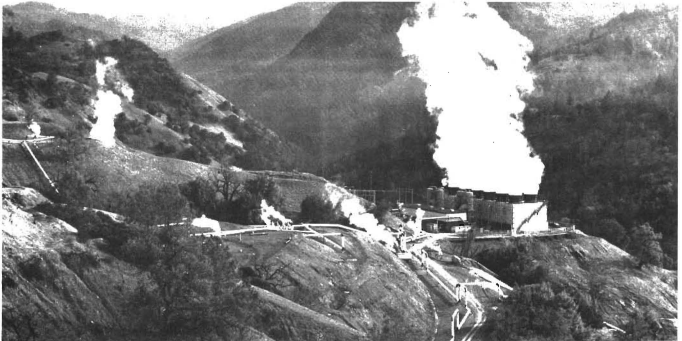
Power plant Units 3 and 4, The Geysers Geothermal field, Northern California. Steam produced from wells passes through the insulated pipeline network to the power plant units.
