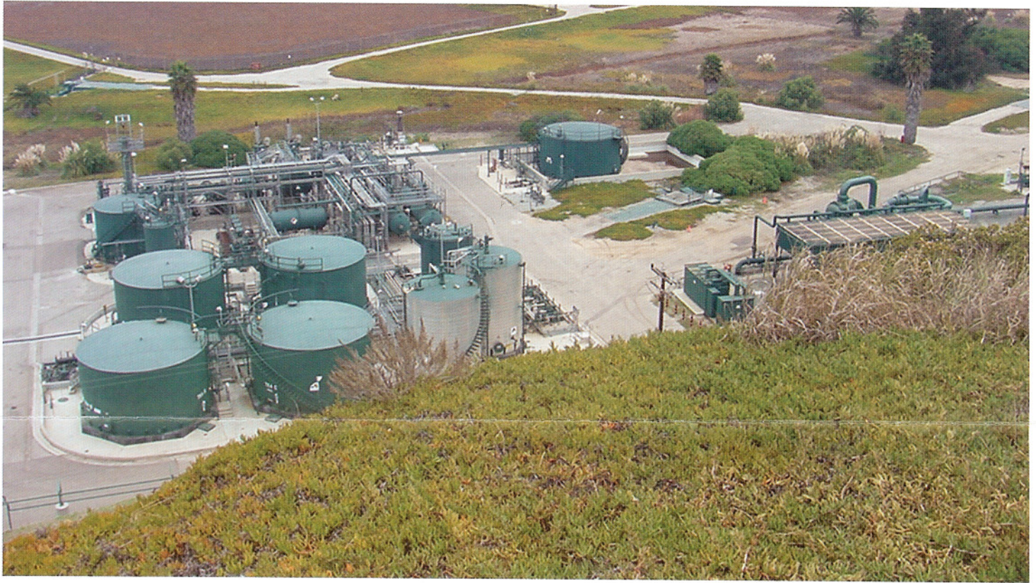
View of part of The Gas Company facility at Playa del Rey.
