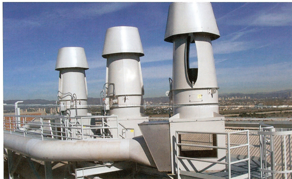
Advanced exhaust fan systems help minimize emissions from natural gas compressors.
