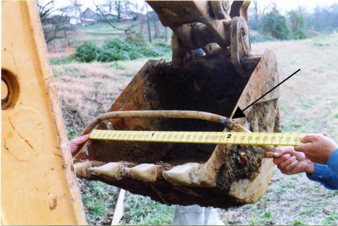
Figure 1. Damaged section of the gas service line to 406 Alabama Avenue. (Arrow shows leak location. Note how the bowed area corresponds with the width of a backhoe bucket.)
