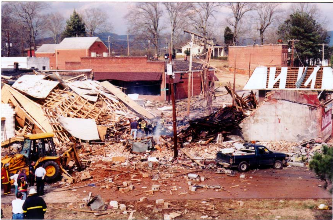
Figure 2. Damage to 404, 406, and 408 Alabama Avenue
