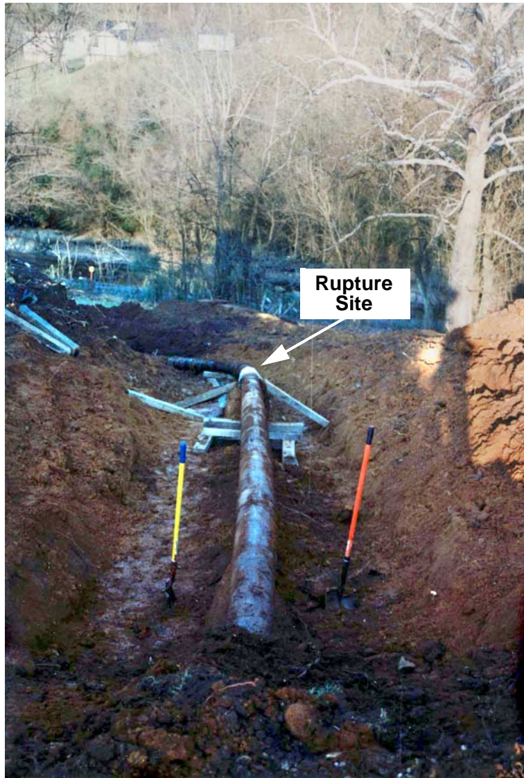
Figure 1. Pipeline on slope showing side bend to the left beyond the rupture.
