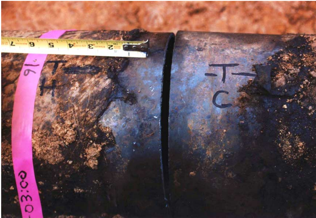
Figure 3. Circumferential crack on top half of pipe with failure initiation region at the 3 o'clock position.
